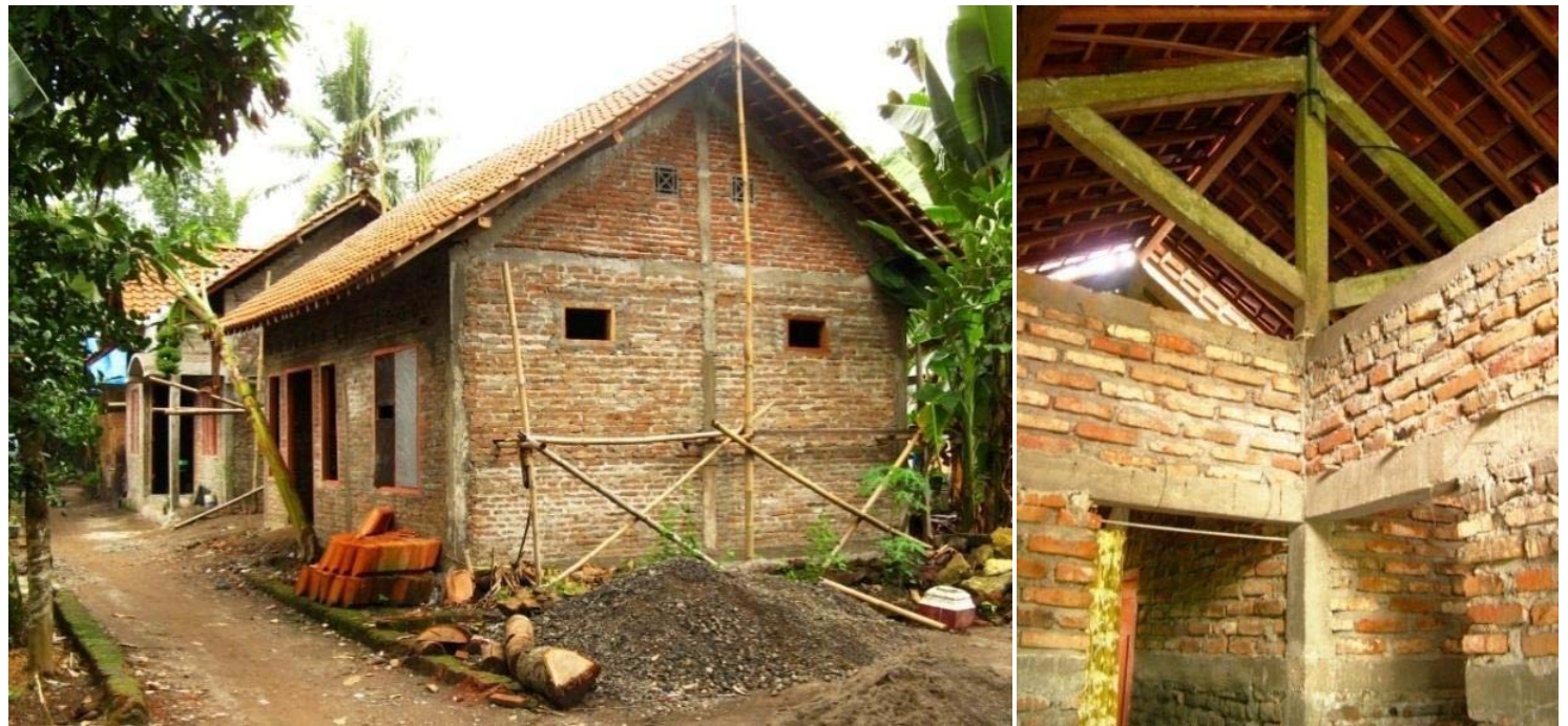
A row of newly rebuilt houses revealing visible concrete frame structures (left) and ring and lintel beams in the interior that follow the recommendations. Pictures taken in early December 2006, seven months after the earthquake, reveal that reconstruction had progressed well ahead of the disbursement of government funding (Jatmika, 2009)
